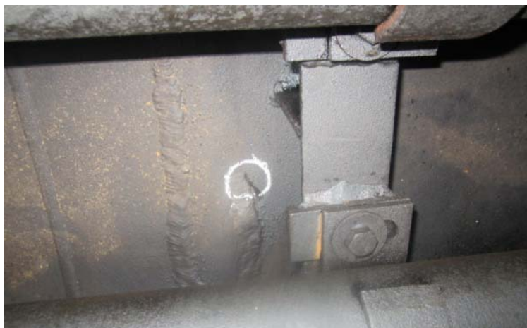
Picture 7. – The cracks spotted from the inside
